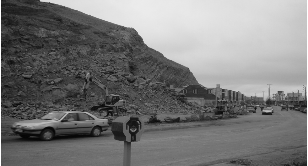
Figure 1: A fault in the city and its destruction on the slopes and effects on the city.
